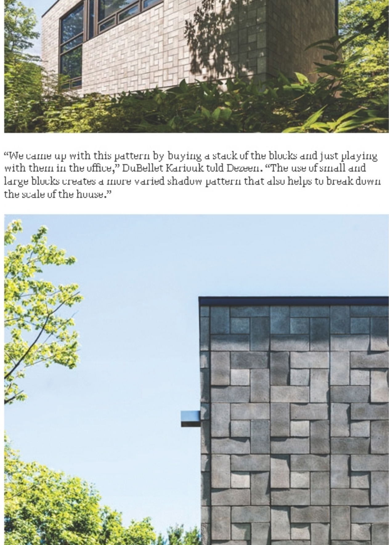
Architect Paul duBellet Kariouk describes the arrangement as a “basket-weave” and it explains how it “takes a very coarse industrial material and makes something graceful out of it.”
